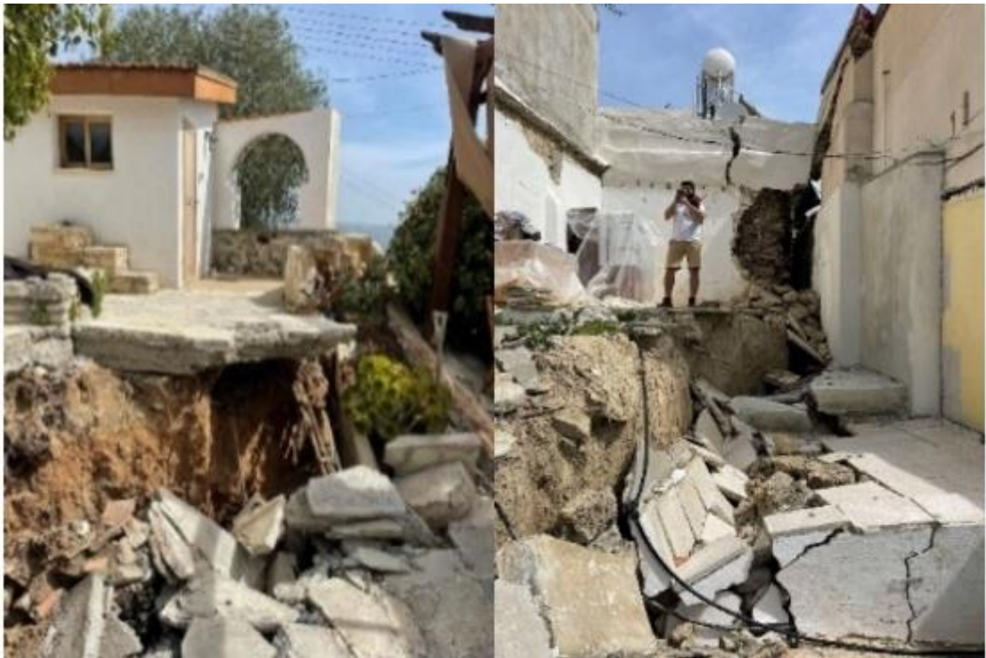
Observed surface and structural damage
